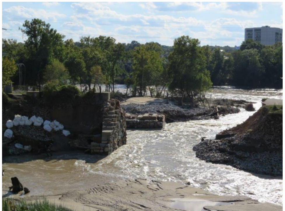
Columbia Canal Breach
