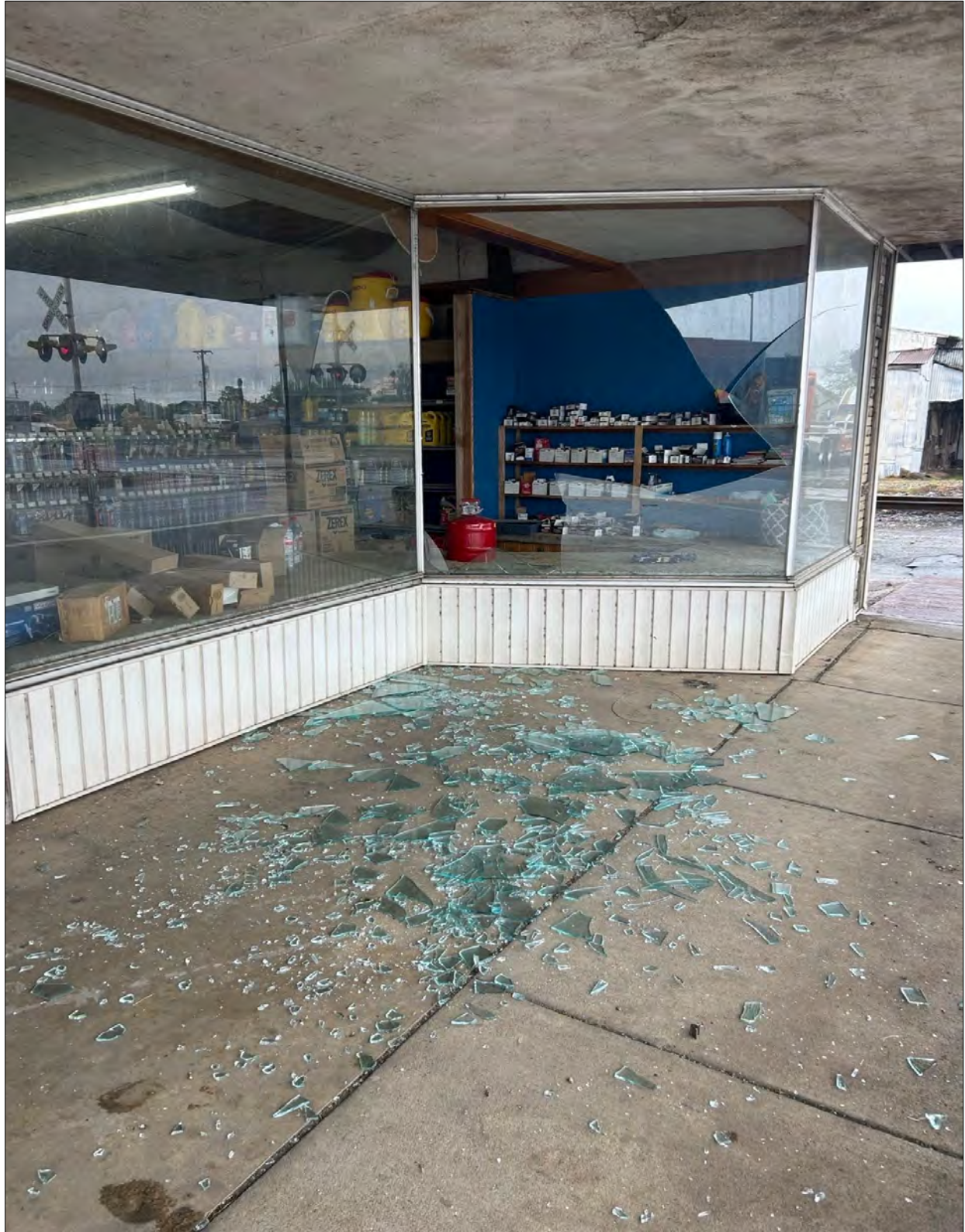
Figure 6: Tornado Damage in Downtown Giddings on April 2nd.
