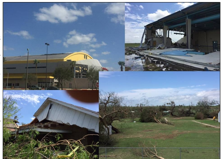
Damage to buildings and trees during the May 31st microburst in extreme southern Hidalgo County, including roof damage at State Farm Arena (top left)
